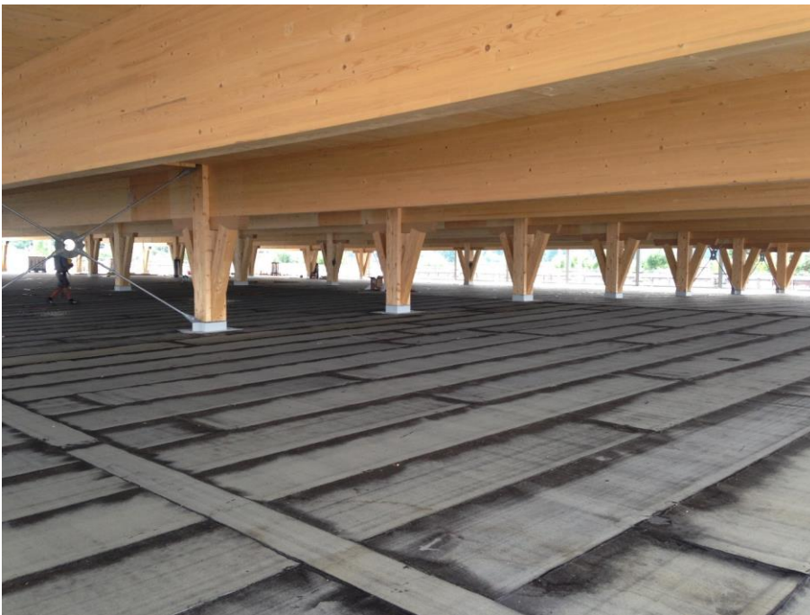
Figure 4: The dimensions of the 5.1m x 15m support grid together with the clearance between the slab joists give a pleasant feeling of space.
