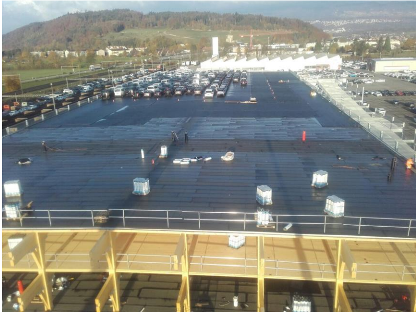
Figure 10: The clients already needs space on the top floor, although construction is still under way.
