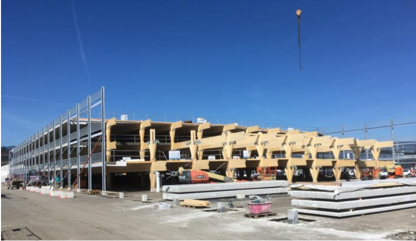
Figure 7: The steel facade pillars can be seen to the left in the picture. All other components are protected from weathering and are made of wood.
