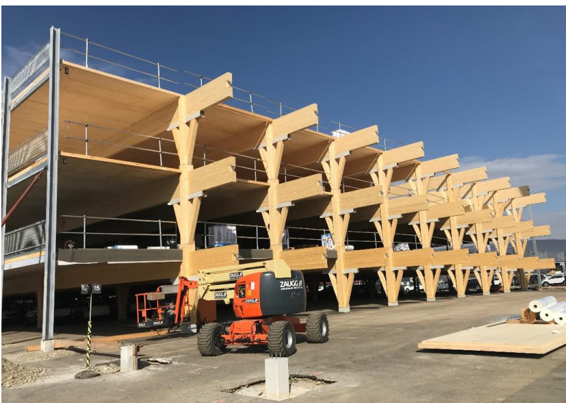
Figure 9: Assembly takes place segment-by-segment across all three storeys. Guardrail are assuring the safety on site.
