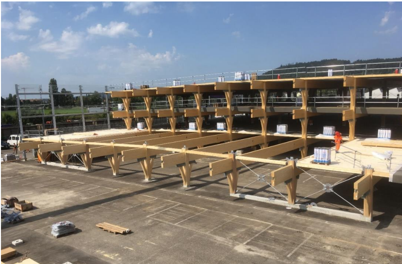
Figure 8: Assembly takes place segment-by-segment across all three storeys. The separation layer and the sealing membrane are fitted immediately after the installation of the carriageway slab.
