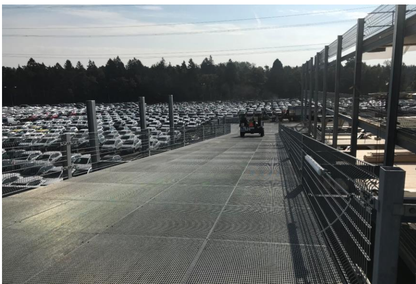
Figure 12: The ramp assures the access of secondary work such as the mastic asphalt.
