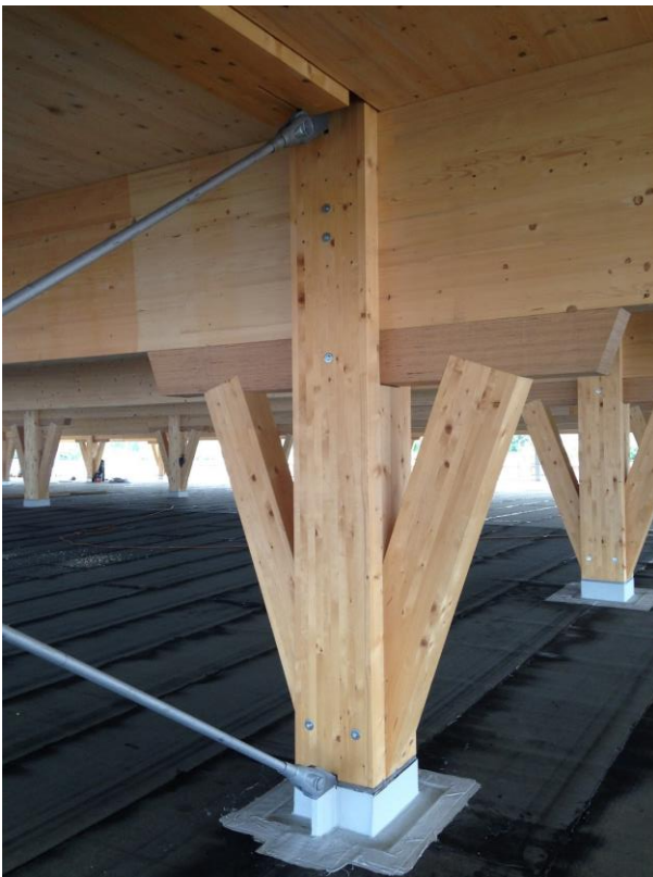
Figure 6: V-form pillars after assembly. The transfer of vertical forces from the upper storeys, from the slab joist, and the transfer of the horizontal forces in the longitudinal and transverse directions at the same point makes this the node point of the car park in the most literal sense of the word.
